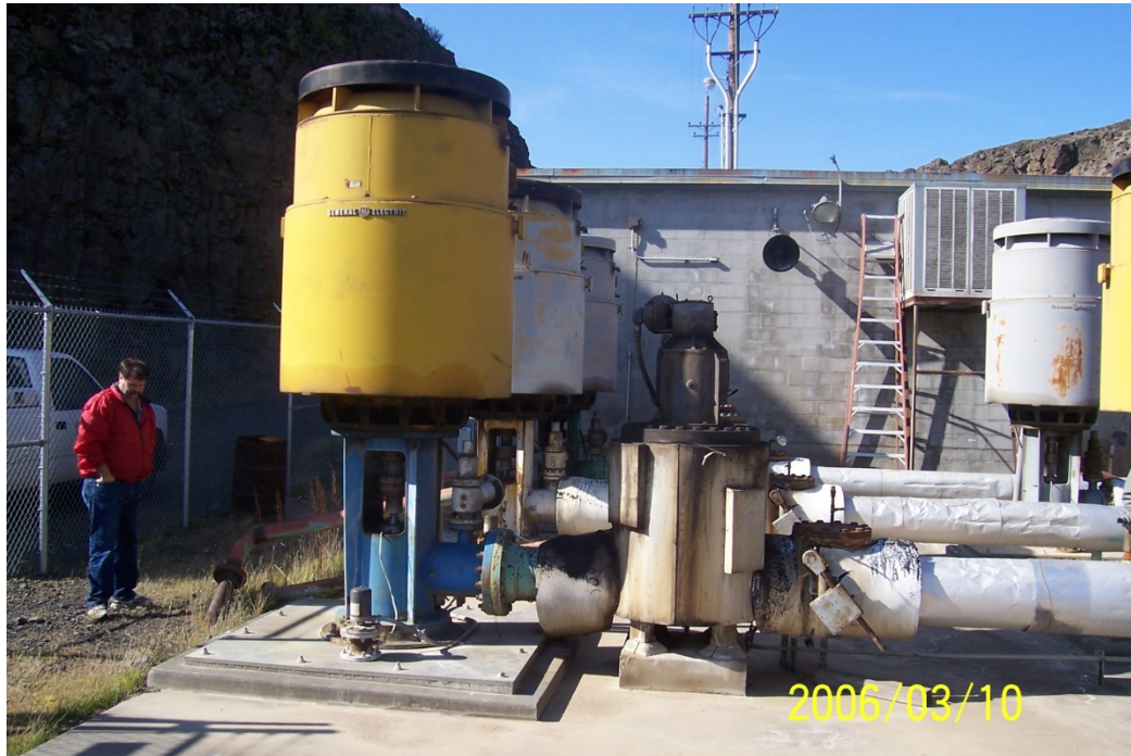
Picture 5-1 – Columbia River Pump Station
